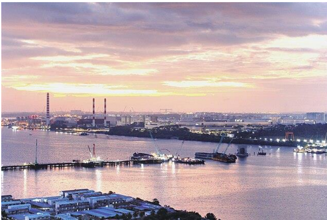
The Johor Bahru-Singapore Rapid Transit System (RTS) Link viaducts under construction in the Johor Strait, March 2023. The bilateral agreement to construct the RTS Link is one of the positive outcomes from past Malaysia-Singapore Leaders' Retreat, and its completion in 2026 will be a tangible symbol of mutually beneficial cooperation that the annual retreat seeks to emphasise. Image from Wikimedia Commons.
